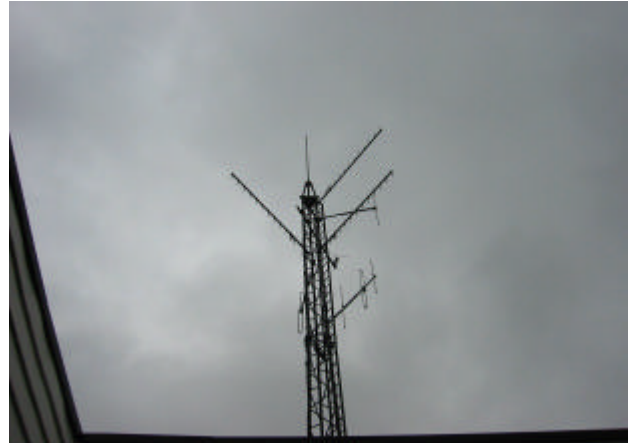
Yagi antenna installed on an ICL Mast at Hertford to establish a benchmark for the Transco PMR system (the lowest antenna to the right side of the mast).
