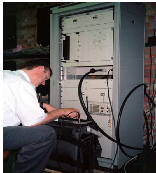
A Radiocommunications Agency engineer inspecting the Tetra base station installation at Didcot.
