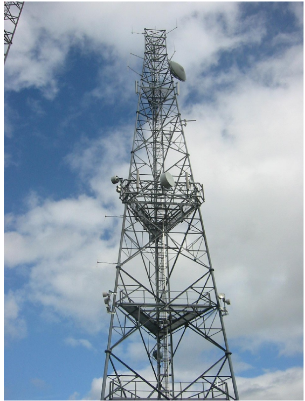
Figure 7 - The mast at Pollnalaght. The UHF co linears are at the top of the mast.
